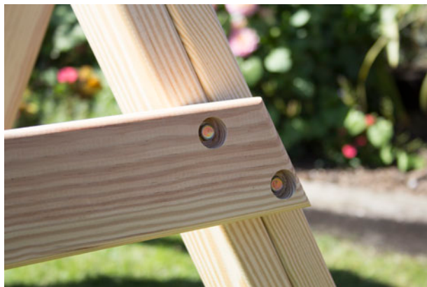
Bottom Brace connection shown
